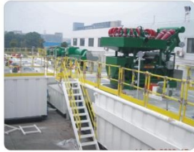
泥浆罐 Mud Tank
