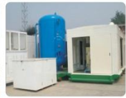
储气罐 Air Receiver
